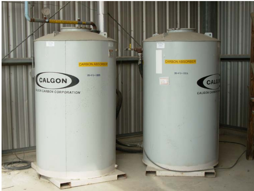
Figure 2 – Dual Canister Carbon Absorber System
