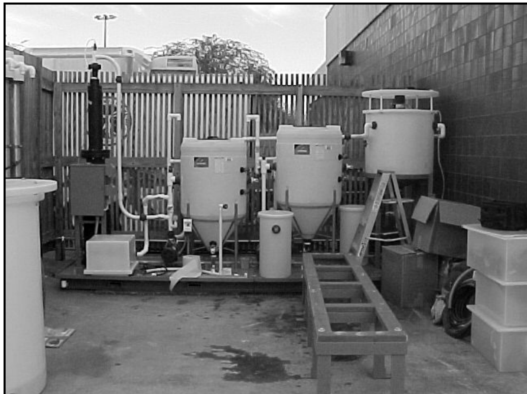
Picture 2 – Leachate Treatment Plant
