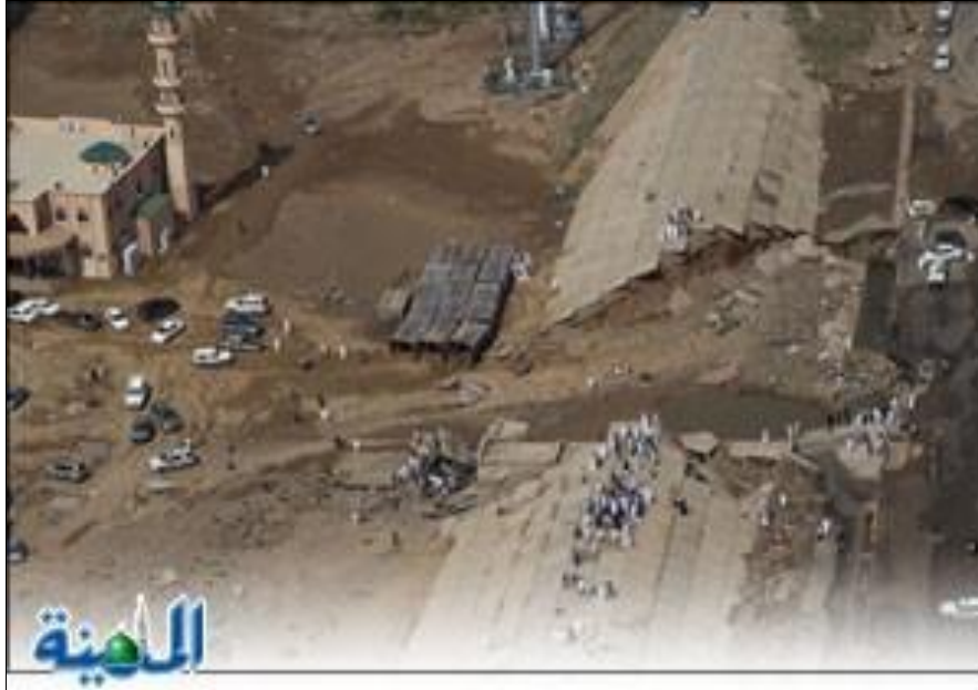
Figure 4.7: Breached Dam near Nakheel (Al-Madinah, 2011)
