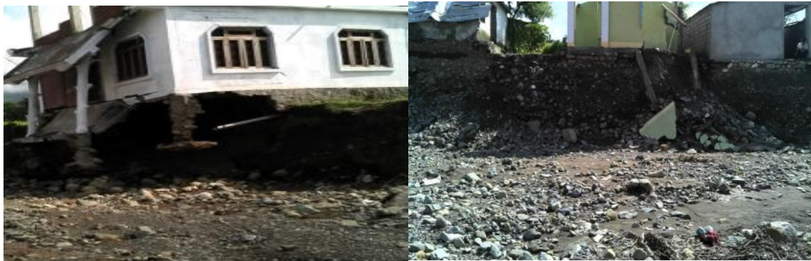
Figure 7. Affected infrastructures from the floods in the Itram River (photo taken by author, 2014).
