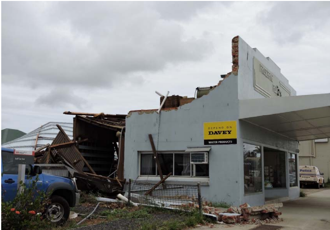
Figure 12. Extensive business premises damage, Proserpine
