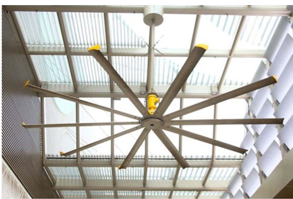
Fig. 2. Activated by human traffic, temperature and humidity, Smart fans will improve thermal comfort levels for residents. (Source: Housing and Development Board, 2014).
