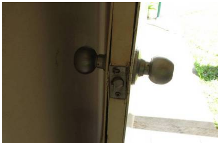
FIGURE 5. TYPICAL LOCK AND DAMAGED DOOR AFTER BEING BLOWN INWARD DURING CYCLONE YASI IN 2011.
