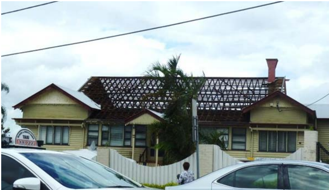
FIGURE 4. FAILED HOUSING AFTER BRISBANE THUNDERSTORMS (NOVEMBER 2014) WITH MISSING ROOFING FROM NOT IMPROVING THE BATTEN TO RAFTER CONNECTION WHEN UPGRADING THE ROOFING TO BATTEN CONNECTION (EXAMPLE 2)
