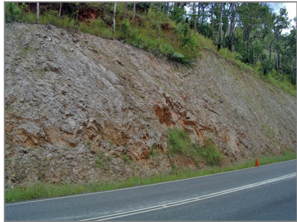
Site prepared for revegetation using hydromulching, Gillies Highway, January 2005 (Photo: Nigel Tucker).
