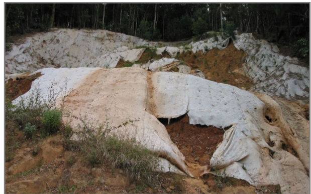
Poor maintenance of geofabric can result in erosion problems, weed invasions and failure of revegetation (Photo: Bruce Jennison).
