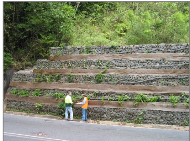
Rock-filled gabions act to retain cuts and fills, allowing steeper slopes, and hence less width of corridor disturbance (Photo: WTMA).
