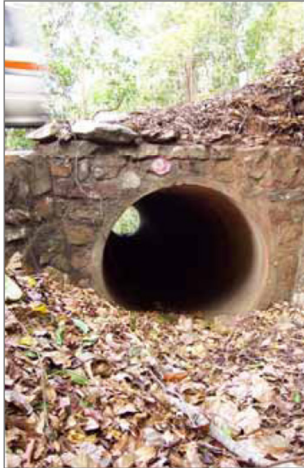
A small existing culvert has the potential for maintaining connectivity across roads for ground-dwelling terrestrial animals.
