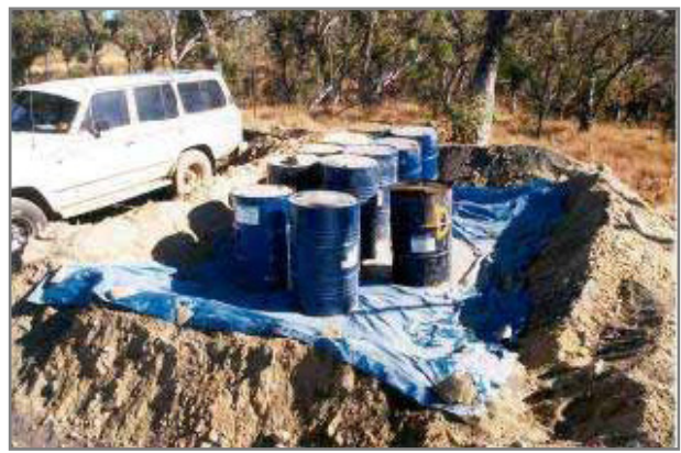
Temporary bunding can help to minimise the impact of road works (Photo: Guy Chester).
