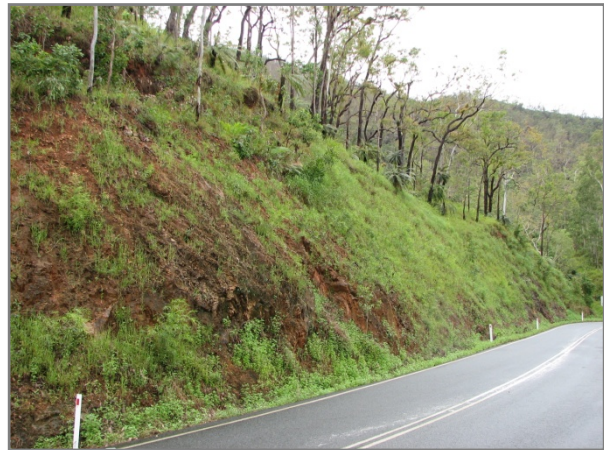
Hydromulching results at the same cutting on Gillies Highway ~ January 2006 (Photo: Nigel Tucker).
