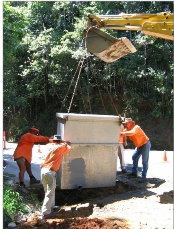
Installation of runoff water treatment system on rainforest highway, northeast Queensland (Photo: Bernd Lottermoser).
