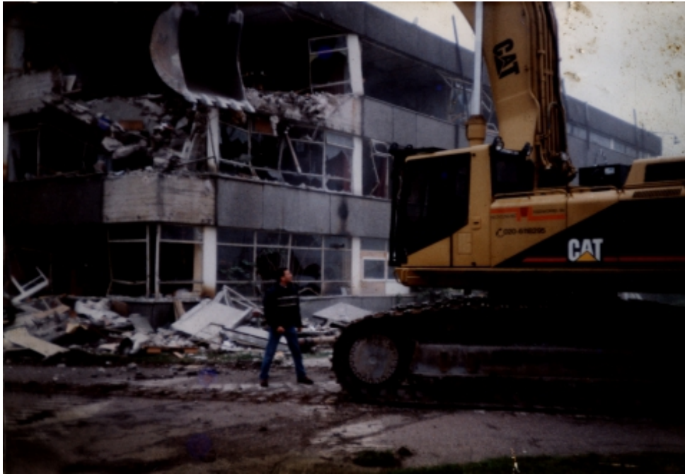
1998: Attempt by the controversial big real-estate investor Luske to evict ADM Free-space demolishing the building with the use of bouncers (source: ADM)
