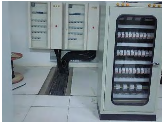
Figure 5 : Power redundancy board.
