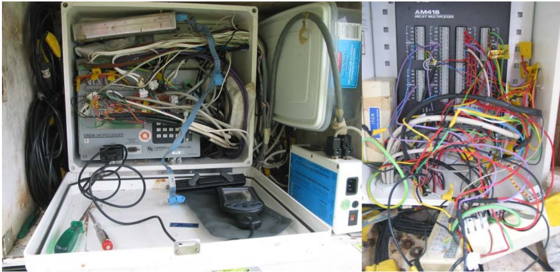
Figure II.5. CR23X-datalogger for automatic data recording (left). An AM416 relay multiplexer is used to increase the number of input channels to the data logger (right).
