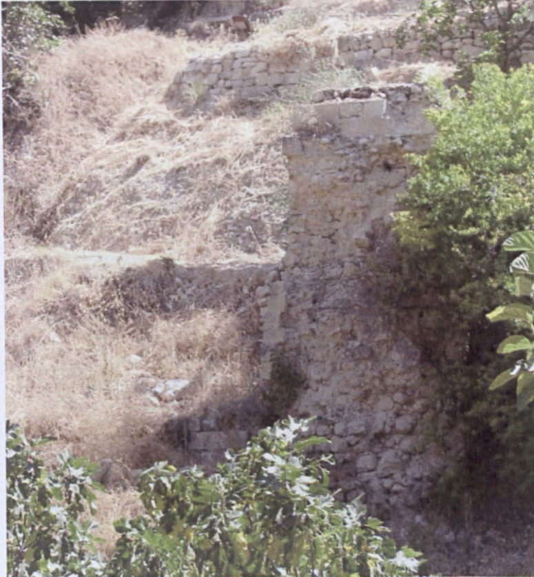
Figure 5. 23. Remains of collapsed penstock, SHU2.
