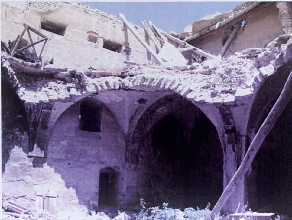
Figure 5. 74. View of collapsed mill house, DAM3.
