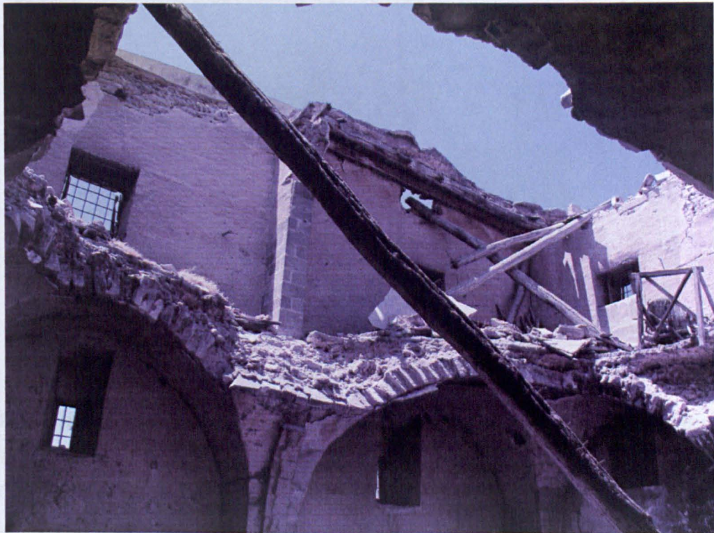
Figure 5. 75. Inside of two-storey mill house, DAM3. The remains of a wooden wheel were located on the second floor.
