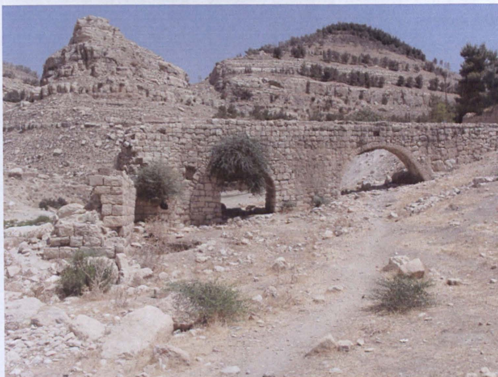
Figure 5. 52. Double-arched millrace with view of collapsed mill house and penstock remains, SK3.
