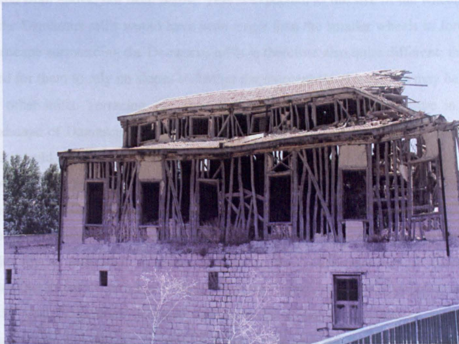
Figure 5. 78. View of facade of DAM5; the modern addition has been constructed over the earlier mill.
