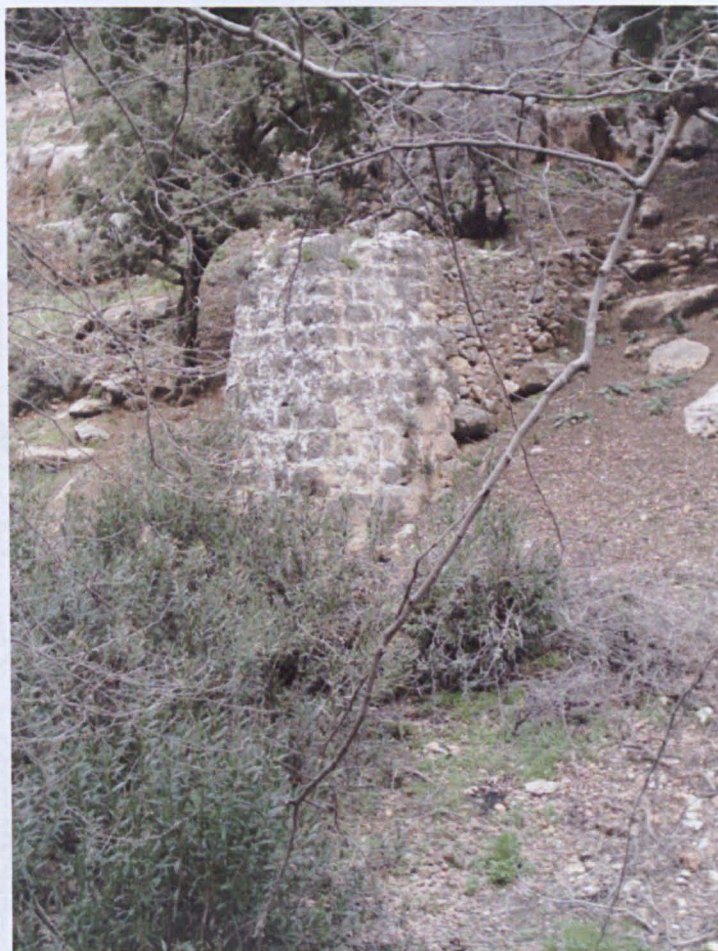
Figure 5. 20. Remains of penstock, RJB4.
