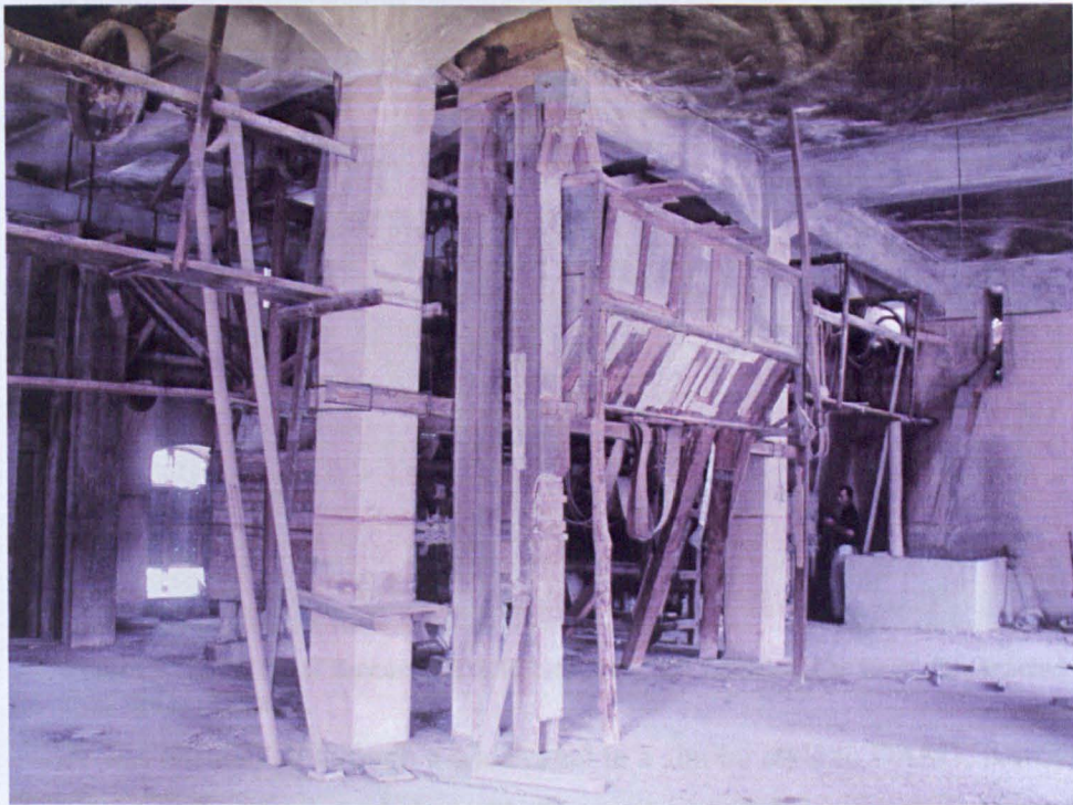
Figure 5. 77. Modern mill room with milling installation, DAM4.
