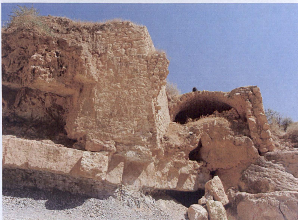
Figure 5. 47. Remains of penstock and wheel chamber, WH10. The structure is resting on bedrock which may have been the cause of its collapse.
