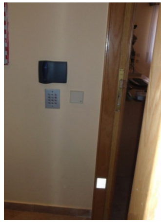
Figure 55 (top left) – Motor to open and close bedroom door. (photo: AC 2008)
