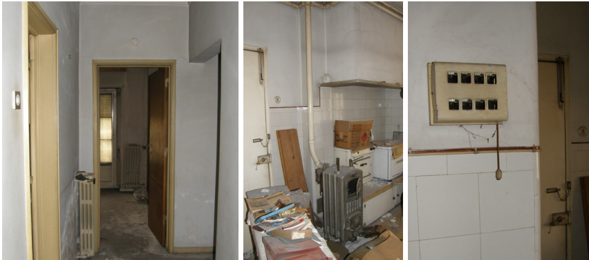
Figure 89 (left) – Wall mounted heating equipment (photo: AC 2009)
