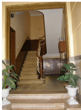
Figures 177 – Left - Water and gas pipes embedded in staircase walls after renovation; Right - original. (photos: SE 2010)
