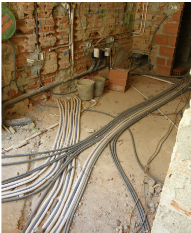
Figure 186 – Screed under-floor ducting. The pre-formed tray is produced from galvanised mild steel and a 12mm plywood cover. (source: http://www.pendock.co.uk/ )
