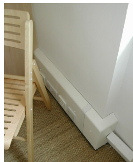
Figure 179 – Multi-compartment casing system for electricity and IC cables. Glastonbury House, London (photo: SE 2004)
