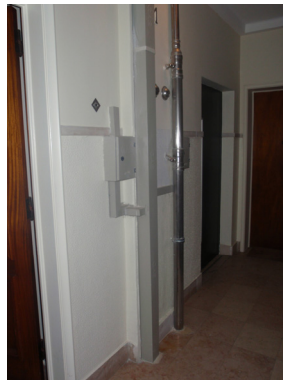
Figures 176 – Left - Electric and telecommunications infrastructure in lobby. Right - Water pipe (surface mounted) and gas pipes (inside metal casing) in staircase after renovation. (photos: AC 2008)
