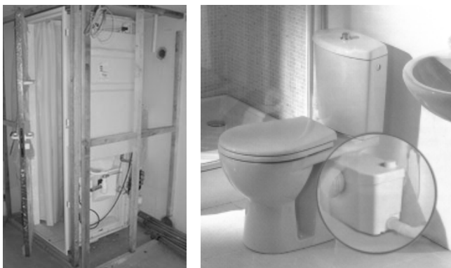
Figure 167 - Prefabricated bathroom in refurbished house (source: http://www.europeanensuites.co.uk/ )
