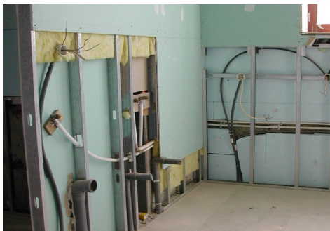
Figure 178 – Pipes and electrical, ICT and domestic cables inside a light construction wall system (frames and gypsum board). (photo: SE 2002)
