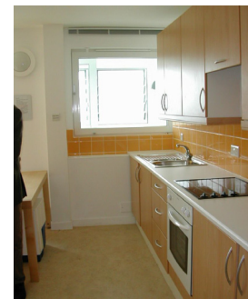
Figure 180 – New lightweight wall parallel to existing wall in order to provide space for cabling and piping. Glastonbury House, London (photo: SE 2004)
