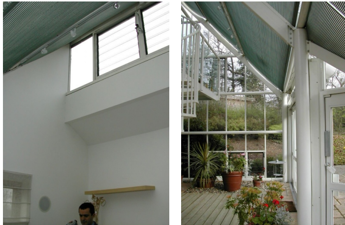
Figures 45 (left and right) – Use of motors to open and close windows to ensure ventilation. Opening and closing actions are activated by readings of wind and humidity sensors, amongst other factors. Millennium House, an Integer project, Watford (photo: SE 2004)
