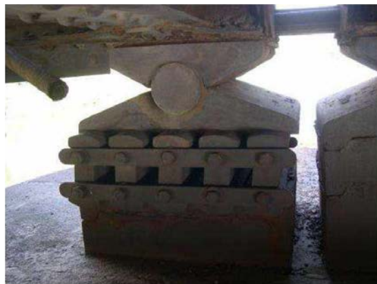
(d) Heavy corrosion in the contact area of support
