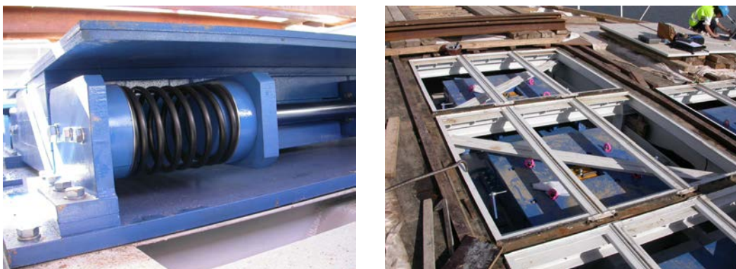
Figure 5.1 Horizontal TMD installed at the mid-span section
