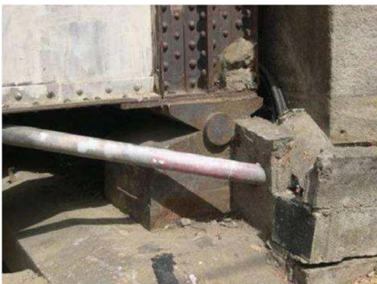
(c) Poor conservation state of the bearings
