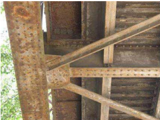
(a) Deterioration in the deck lower elements
