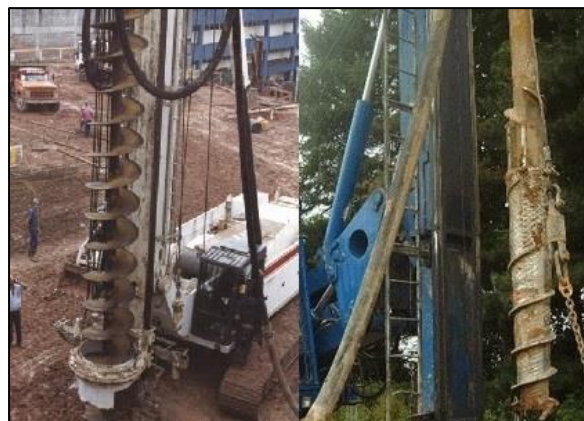
Figure 4.2 – On the left, a photo of a CFA pile and on the right, a photo of a OMEGA pile
