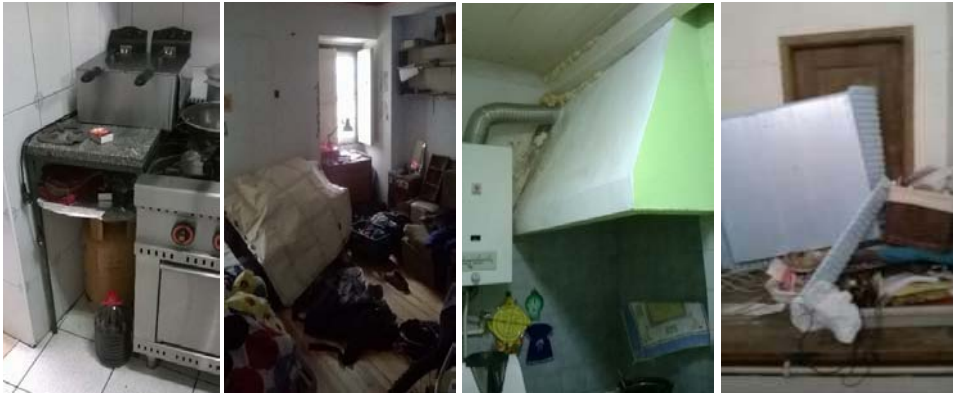
Fig. 5. Examples of fire safety problems found within the old town buildings
