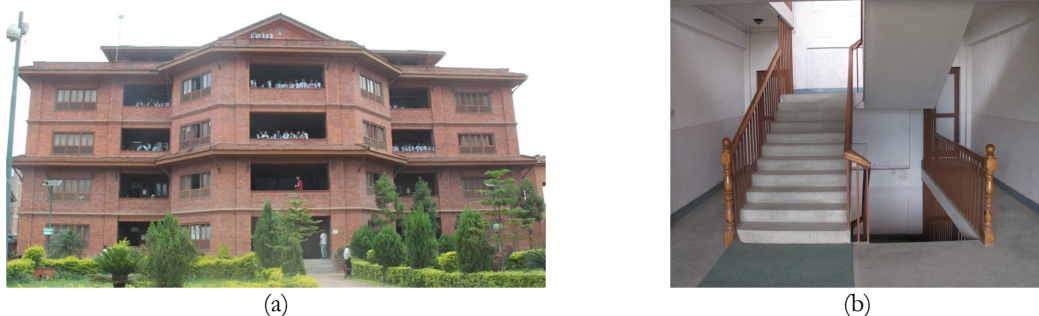
Figure 3.22 – WD1 building observed in the course of field survey; (a) and (b) No structural damage and insignificant or hair line cracks on few infill panels
