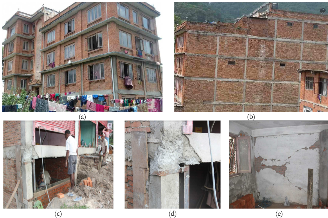
Figure 3.18 – MRT2 building scenario observed in site survey; (a) East-South elevation, (b) North elevation, (c) and (d) Repair and maintenance works on the beam-column joint and (e) Diagonal cracking on infill panel
