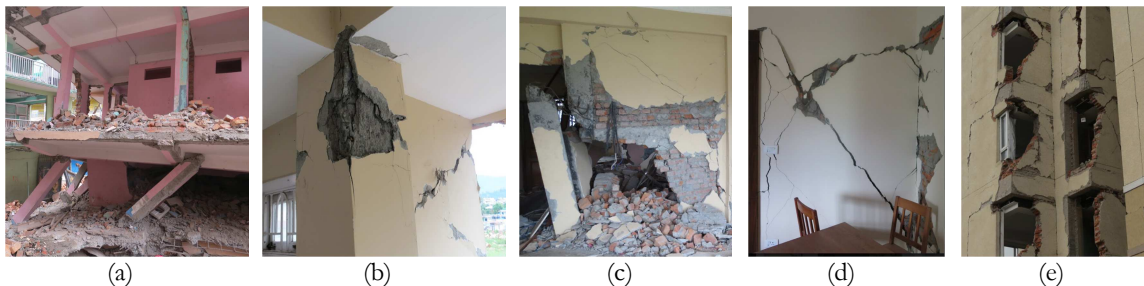
Figure 1.2 – Examples of infill wall negative contributions on infilled RC buildings; (a) Soft-storey, (b) Shear in column, (c) Short-column, (d) In-plane and (e) Out-of-plane failure of infill walls
