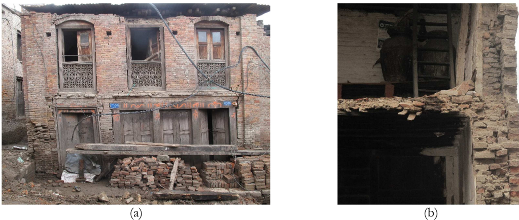
Figure 2.15 – Earthquake damages and failure modes; (a) concentration of the damage in the ground floor due to the openings disposition and (b) Total collapse of the building's façade due to the inadequate anchorage of the floor diaphragm to the wall
