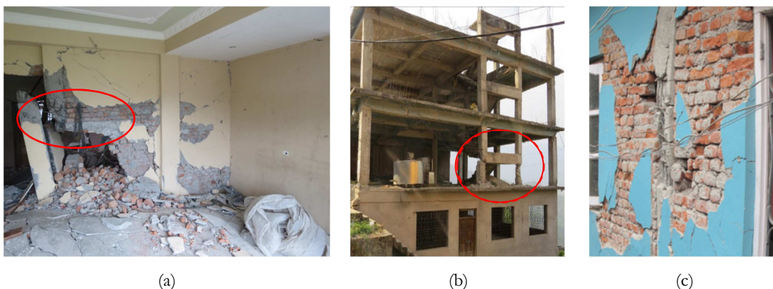
Figure 2.4 – Examples of short-column failure due to the existence of (a) Staircase landing and infill, (b) Stair landing beam and (c) Infill panels with openings
