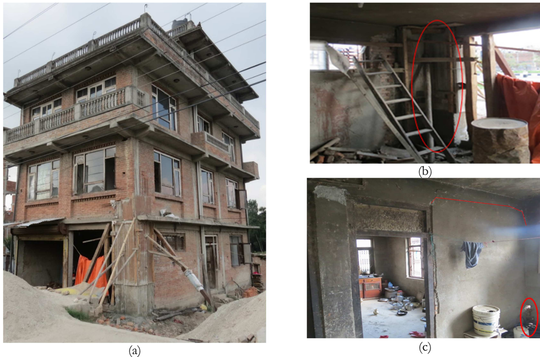
Figure 3.10 – CCP2 building during the site inspection; (a) Geometrical 3-D view, (b) Maintenance work on damaged corner column and (c) Crushing of infill panel and separation of infill panel at the beam interface
