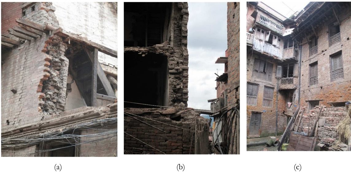
Figure 2.12 - URM buildings construction details; (a) Masonry wall leafs disposition, (b) Connection between the timber floor and the transversal wall and (c) Buildings block
