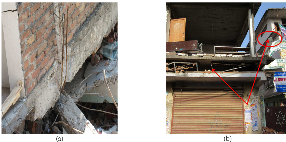
Figure 2.6 - Failure caused by weak beam-column joint; (a) Poor beam-column reinforcement detailing and (b) Pancake collapse
