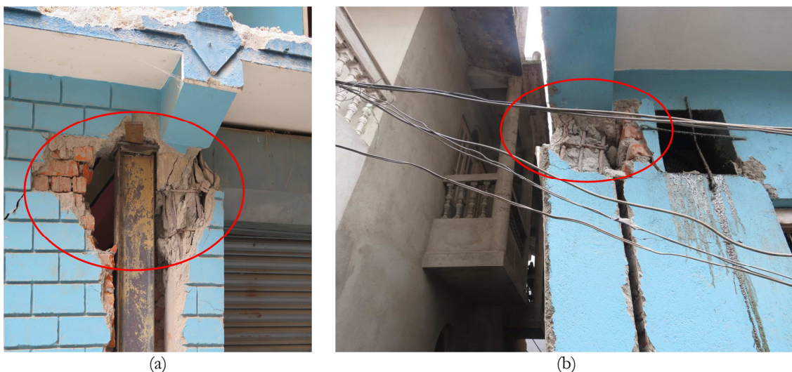
Figure 2.9 – Examples of shear failure at top of column induced by masonry infill panel; (a) Initiated by the strength difference of the adjacent column and (b) Shear failure at the corner column
