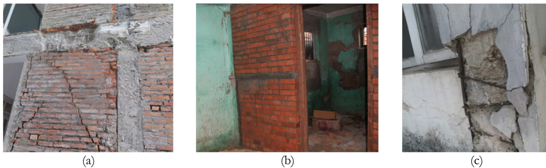
Figure 3.2 – Typical state of structural and non-structural elements observed during visual inspection; (a) Diagonal cracking, corner crushing and shear cracking on the infill panel, (b) Construction of new infill panel on the open ground storey and (c) Poor concrete quality, poor stirrup spacing and its distribution, and poor concrete compaction
