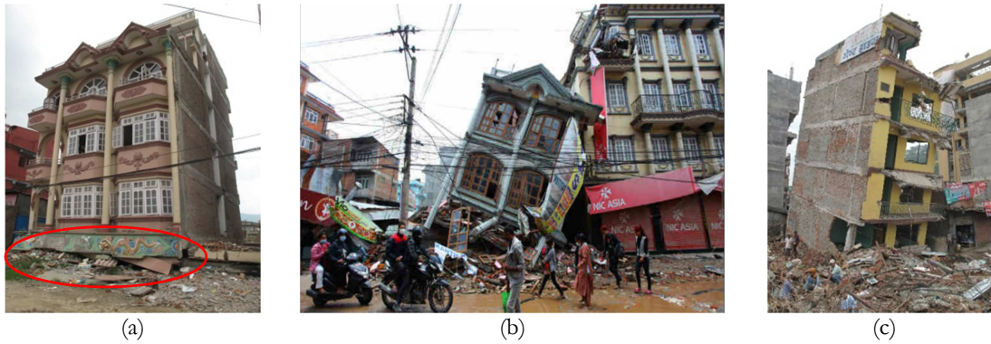
Figure 2.3 - Examples of buildings subjected to soft-storey collapse during the Nepal earthquake; (a) and (c) Building collapsed due to soft-storey at the ground floor and (b) Soft storey followed by pounding
