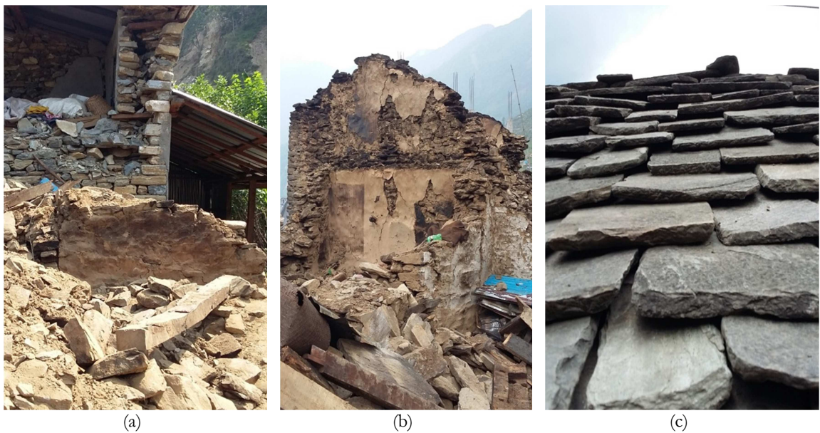
Figure 2.16 - Typical features of rural buildings; (a) Heavy dry stone masonry wall, (b) Two-storied building subject to in- and out-of-plane collapse and (c) Heavy roofing stones
