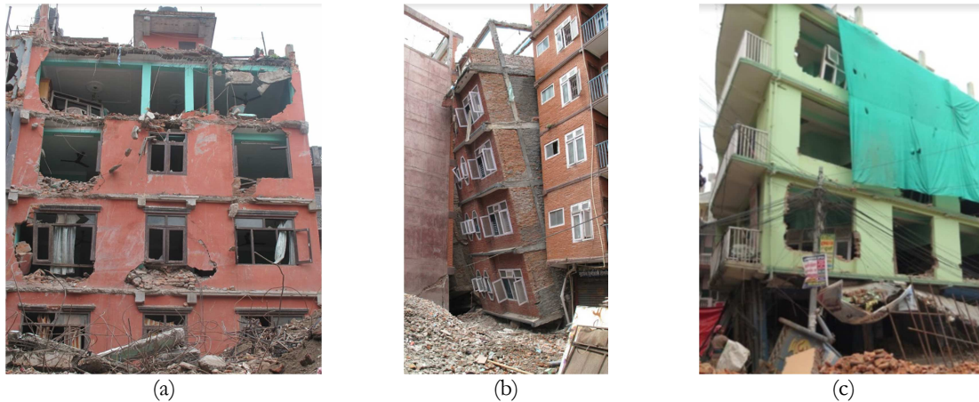
Figure 8.1 – Representative damaged buildings due to the distribution of infill walls observed after Gorkha earthquake; (a) Total in-plane crushing of the infill walls, (b) Soft-storey building along with pounding mechanism and (c) Soft-storey mechanism and out-of-plane failure of the infill walls
