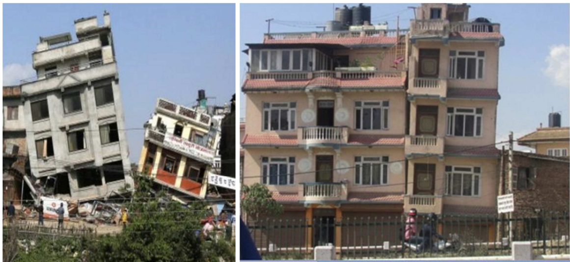
Figure 2.5 - Examples of buildings failure; (a) Pounding followed by soft-storey and (b) Interaction between the buildings due to lack of seismic gap
