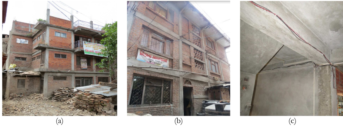
Figure 3.6 – CCP1 building recorded during the reconnaissance after the Gorkha earthquake; (a) and (b) North and South facing, respectively, and (c) State of infill panel and frame elements and their connections
