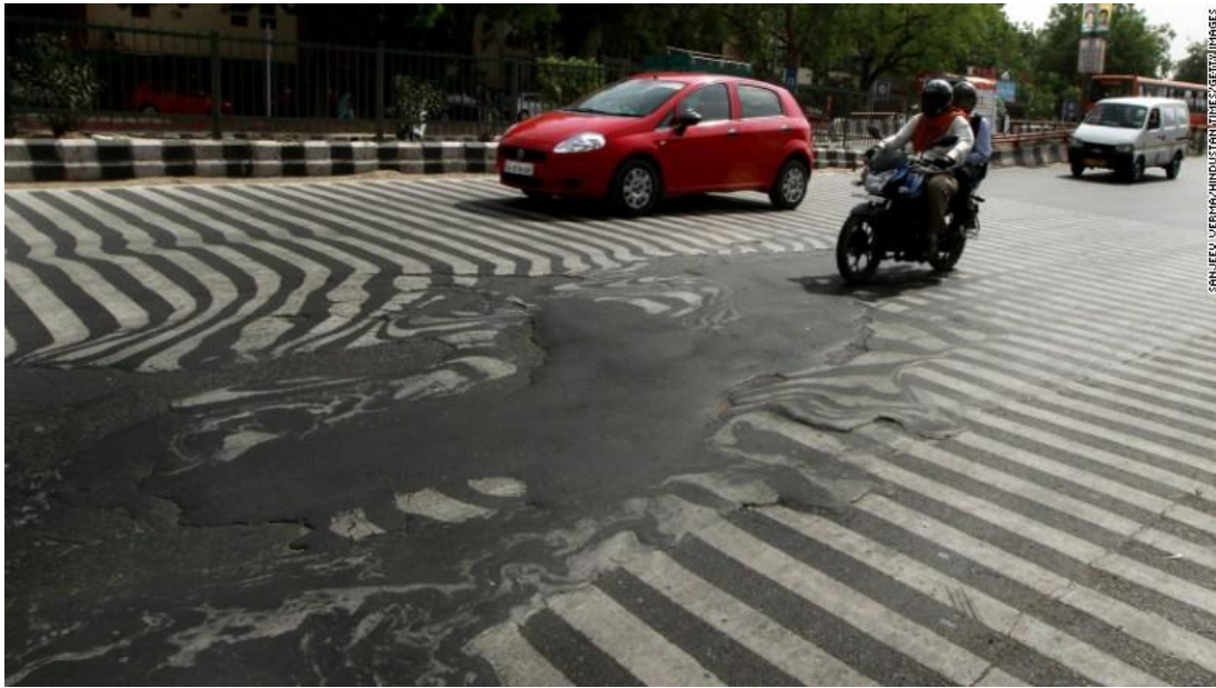
Figure 7-15 Some of the roadways in India are melting because of the recent heat waves that hit the regions
