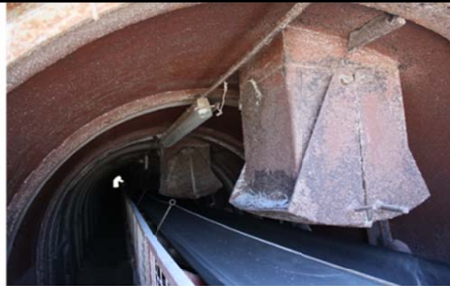
Shutters in the tunnel roof allow material to fall onto a moving belt by gravitational forces (opening size can be adjusted to modify rate of flow)
