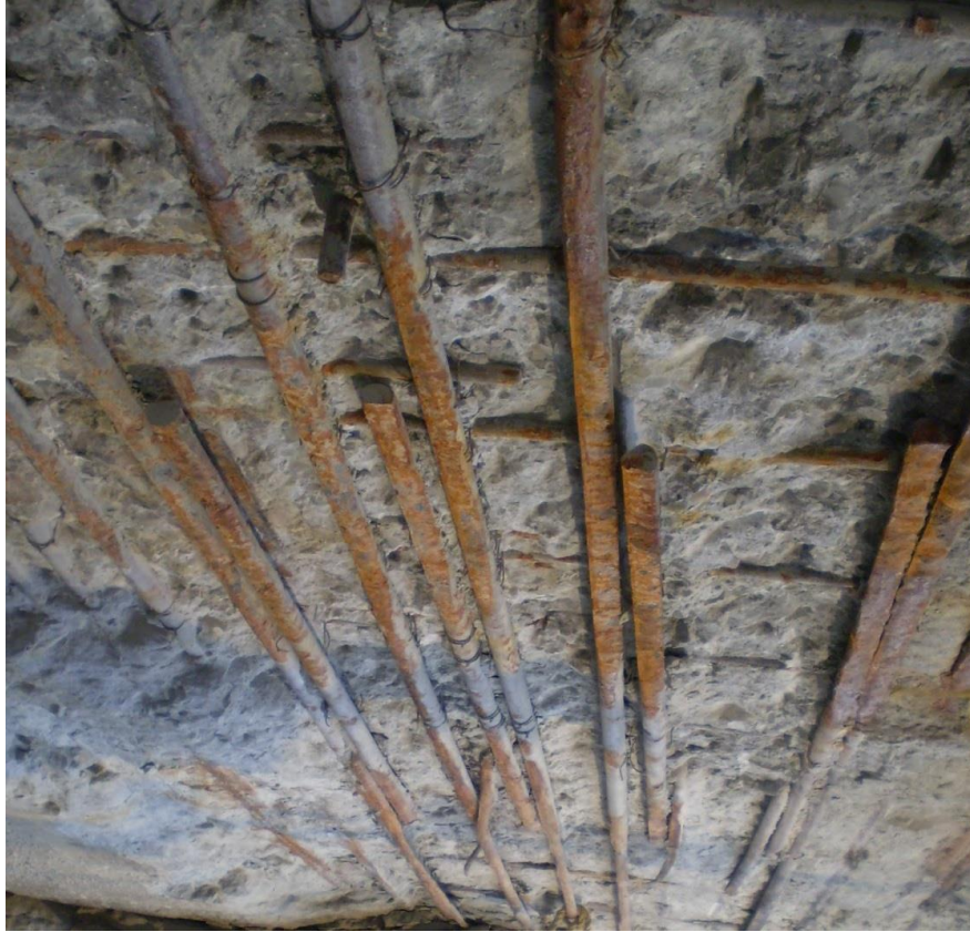
Figure 1-1 Corroded steel reinforced concrete beam ( www.adbengineering.com ).
