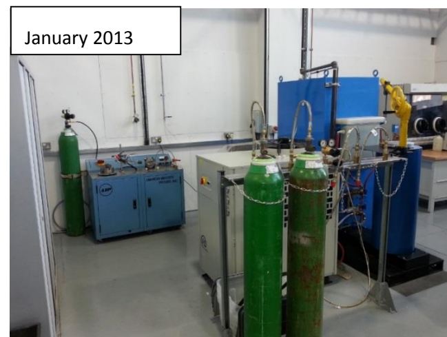
Figure AI.1 Images showing the installation of AIP 6-30H in the Quarrell laboratory, The University of Sheffield
