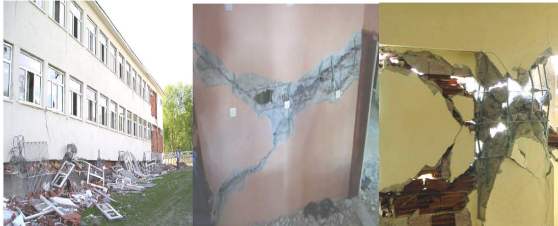
(a) Collapse due to soft storey (b) Shear wall failure (c) Brittle column failure
