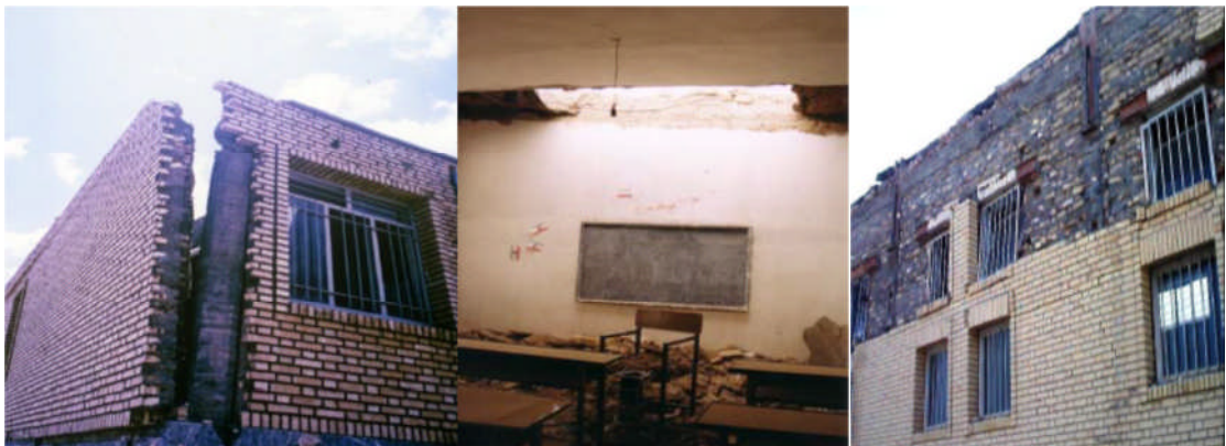
Figure 2.2 – Lack of integrity in school buildings in Iran (SRO 2011)
