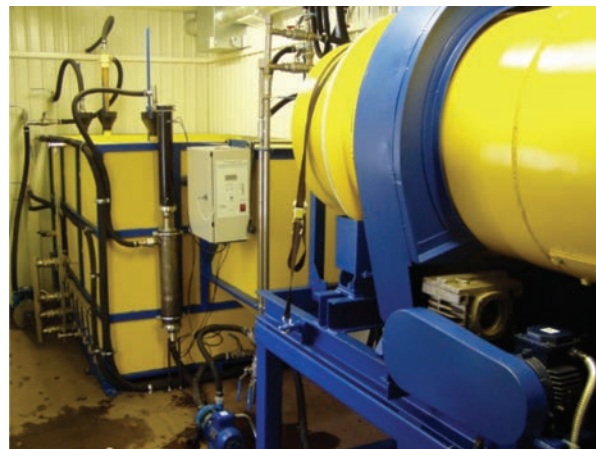
Fig. 9. Mobile complex of ultrasonically assisted galvano-coagulation wastewater treatment. Placement of equipment inside the container
