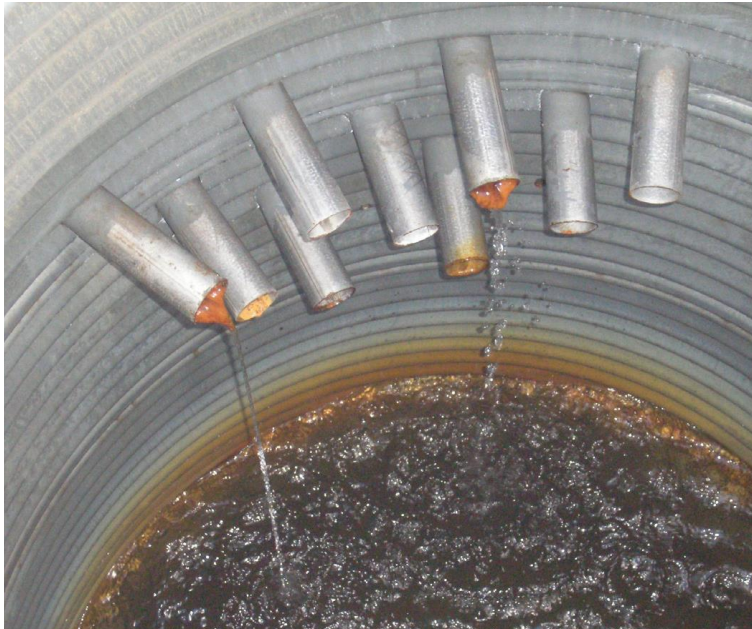
Fig 1 – Example of sub-horizontal drain outlet, where partial clogging of several pipes can be observed.
