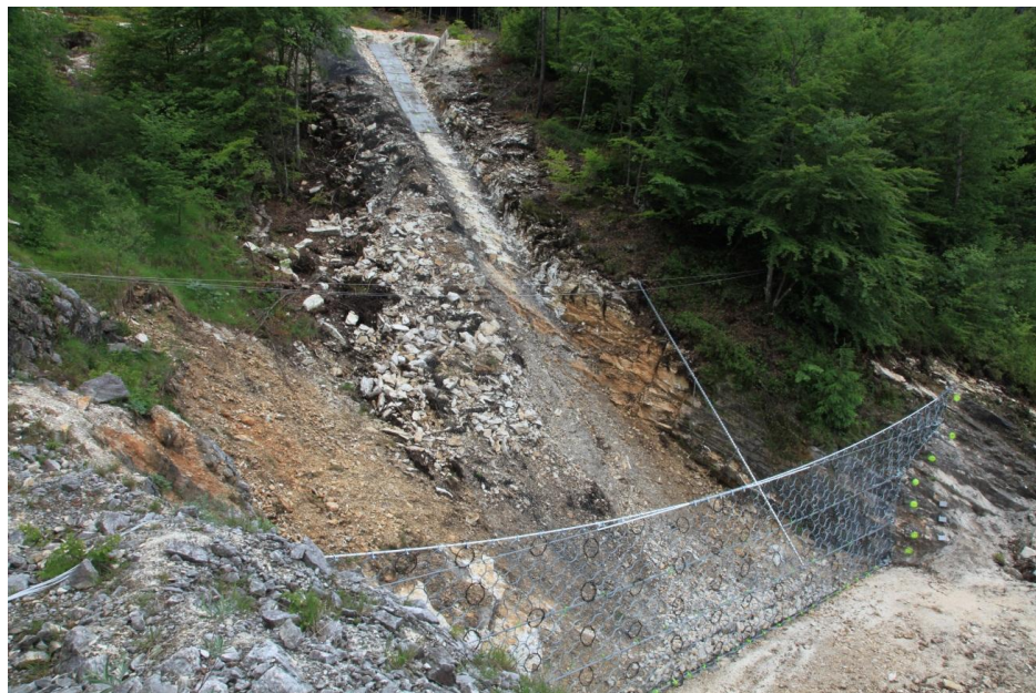
6 7 Fig. 4. Example of a debris flow barrier (installed at the Pieve di Alpago (BL, 8 Italy) test site, see Section 4 ).
