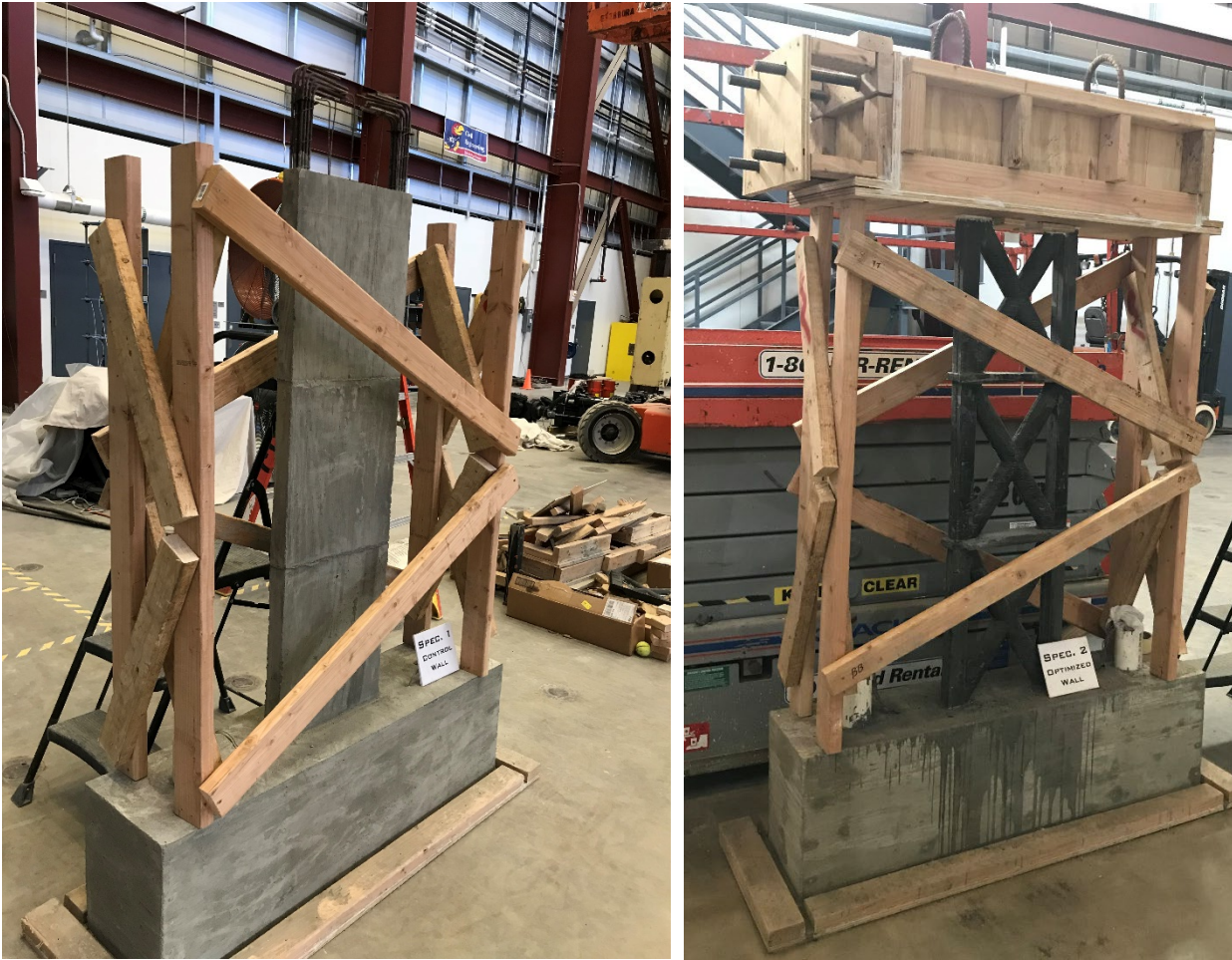
Figure 3.10: Support structure/falsework and formwork for top block in control (left) and optimized walls (right)
