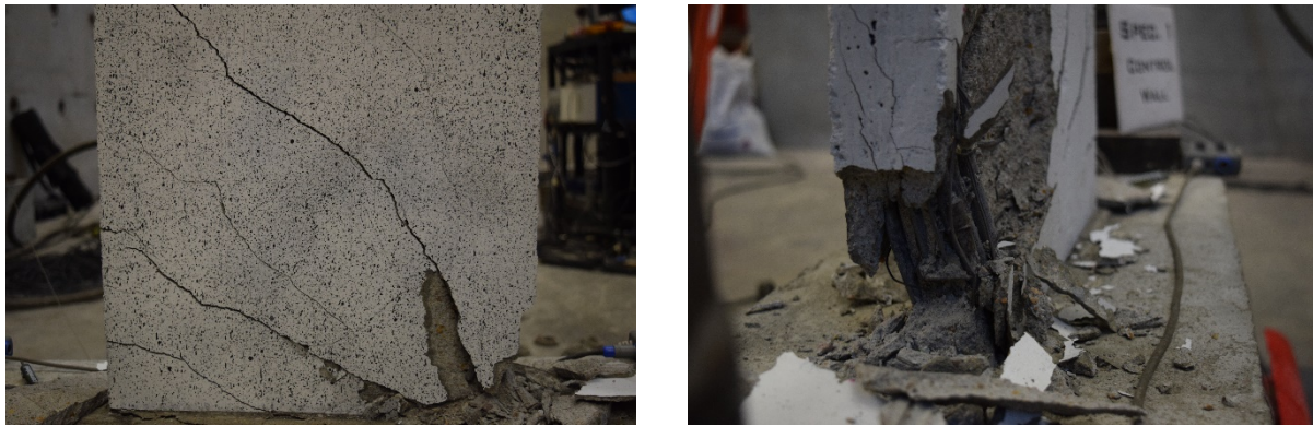
Figure 4.8: Control wall damage at failure
