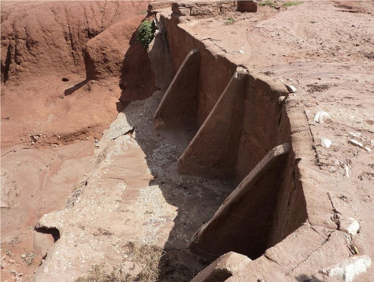
Figure 10. Gully erosion near Taita Sisal Estate reservoir, close to Mwatate town. A brick barrier was constructed to prevent the sediment from flowing to the sisal estate dam, but it has now reached its full capacity. (Hohenthal 5.2.2013)
