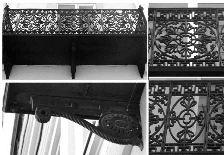
Fig. 2. Balcony fencing and balcony bracket on the building number 2 at Starozamkova Street (1732)
