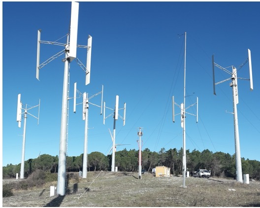
Figure 1.19: Ropatec TS30 wind farm near Volterra, Italy [Ropatec, 2013].
