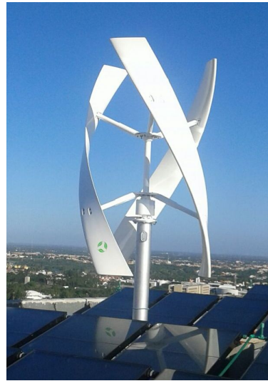
Figure 1.22: UGE Visionair 3 (1KW rated power) in a roof in Brazil [UGE, 2016].
