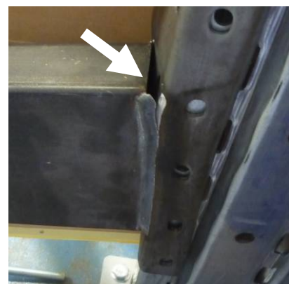
a) Component: Weld Test: 130/250-1352B Failure of Weld
