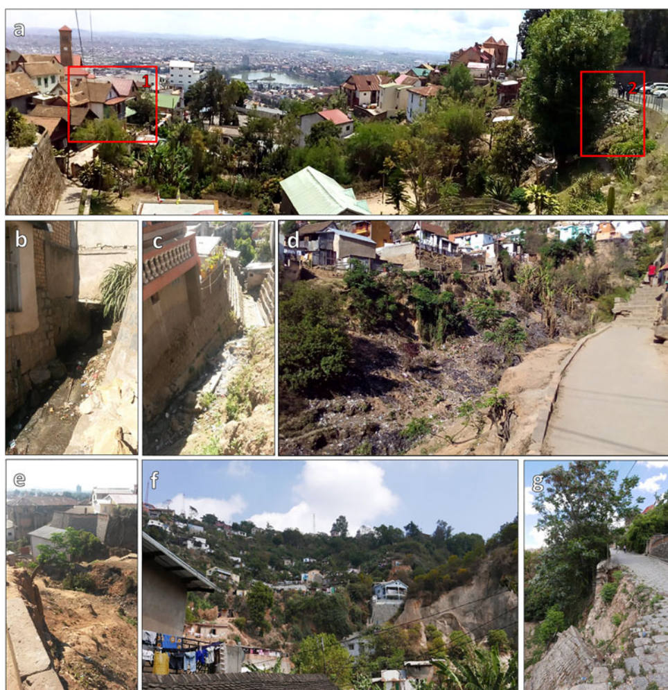
Figure 12. Geomorphological-erosional problems in basins 3–4. Hanging-like valley (a); damaged buildings (red square 1), retained roadway slope (red square 2). Creek 3 hydraulic narrowing (b). Creek 4 lavaka-like gully erosion (c) and hovels built within the creek bed (d). Basin 25 urbanization (e). Source: Author
