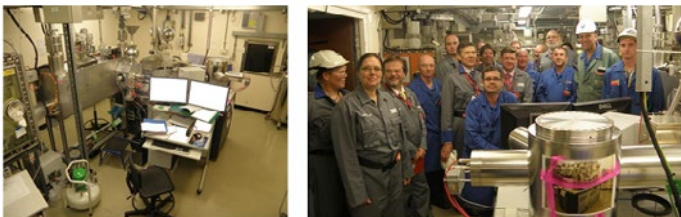
Figure 4. Triton connected to glove box (left) installed in the OSL and photo of the inauguration (right).
