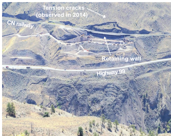
Fig. 4 Front view of the 10-mile Slide. Photo taken in July 2016
