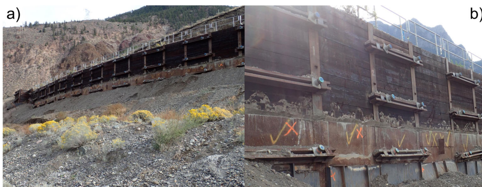
Fig. 9 View of the retaining wall from the northernmost area of the landslide (a) and close view of the anchoring system (b)
