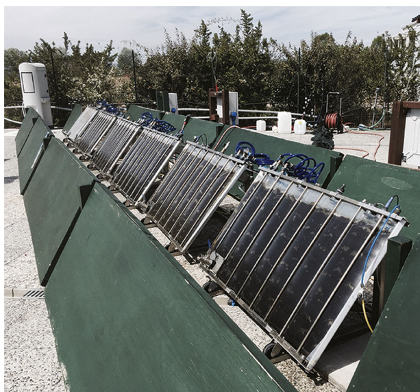
Figure 1. GWPP ® -III reactors installed at the experimental area of Fotosintetica & Microbiologica S.r.l. (Sesto Fiorentino, Florence, Italy). Dummies are placed in front, back, and sides of the reactors to simulate a full-scale plant. The panels face south with an inclination of 50°. The distance between rows is 1 m.
