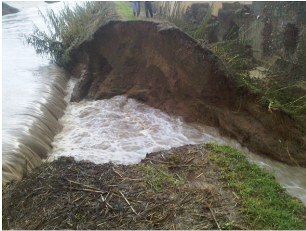
Figure 1 Levee failure in the Ombrone Pistoiese river (Tuscany, Italy) induced by seepage during the flood event of 25 December 2009. Photo by Land Reclamation Authority of Ombrone River.
