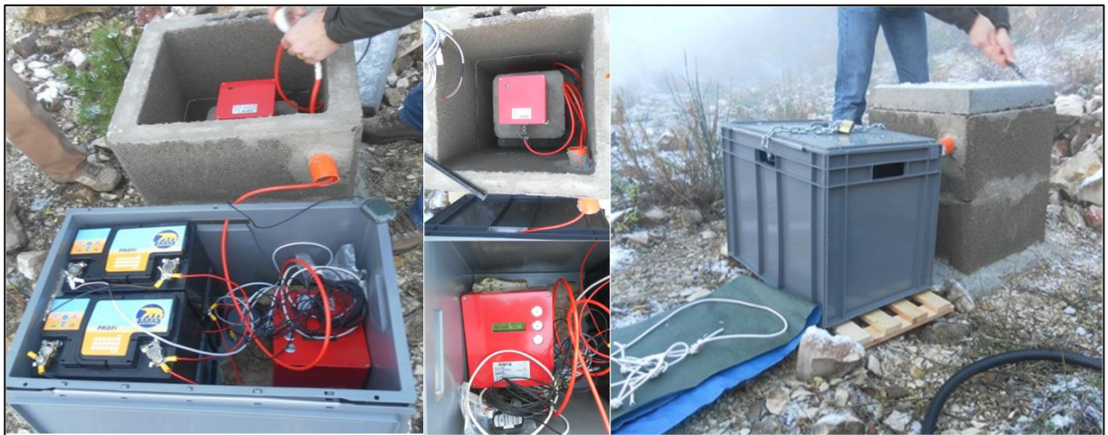
Figure 12 – Visualization of one of the four seismic stations. The grey box contained digitizer and electrical battery supply, sensor was settled on a concrete base protected from the outside by means of a reinforced manhole.
