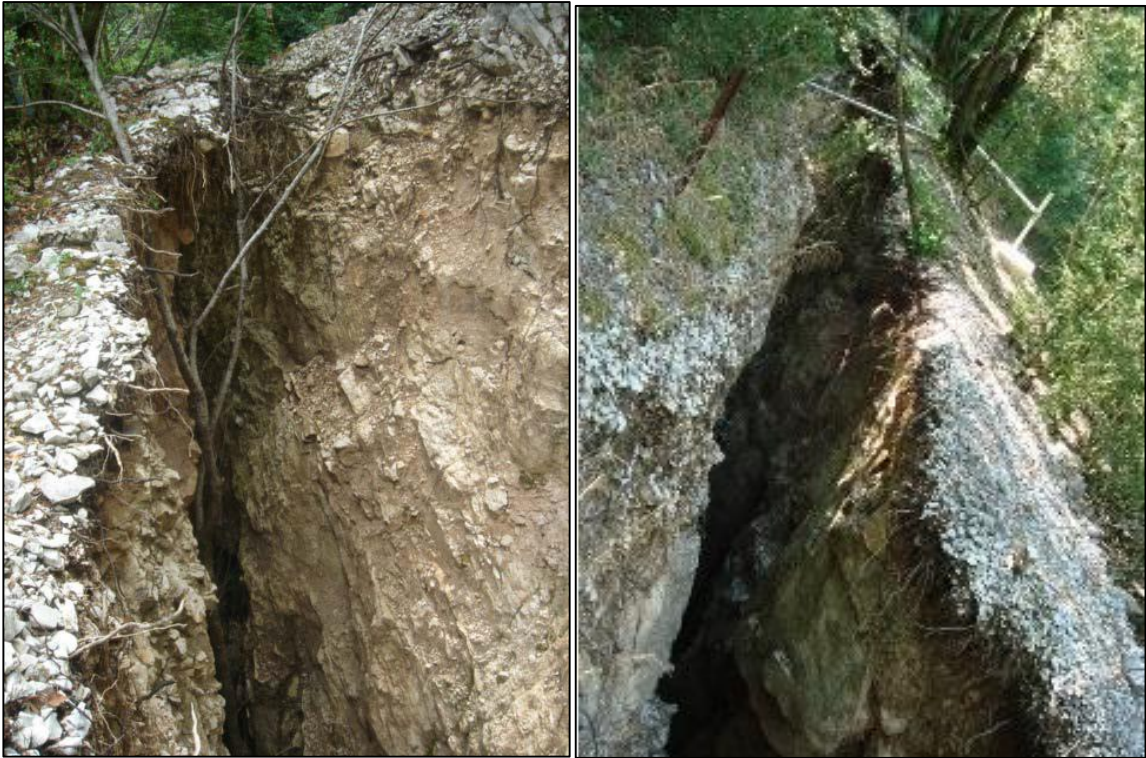
Figure 9 – Details of the main tension crack (upper boundary) on the rear side of the quarry.
