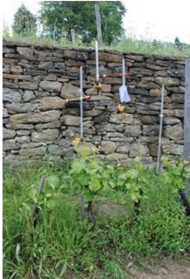
figure 5: piezometers installed on the monitored dry-stone wall to measure the water level behind the wall itself
