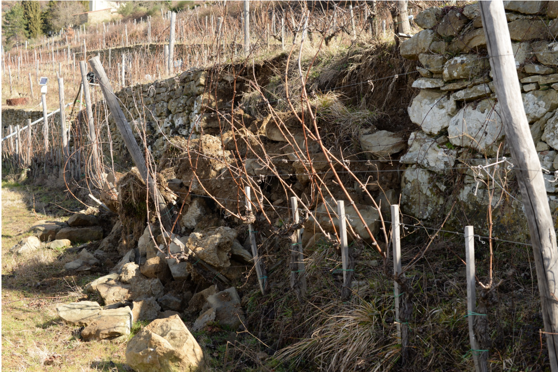
figure 2: example of dry-stone wall collapsed after intense rainfall
