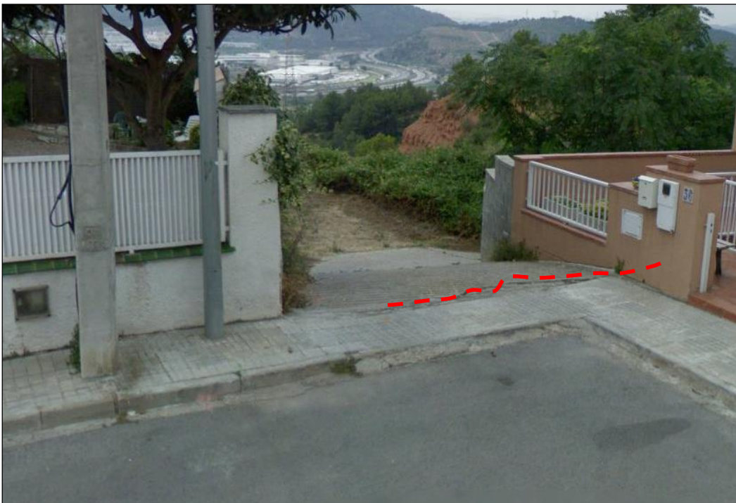
Figure 122: Image of building conditions. In correspondence of PS were found fractures along the road and the walls surrounding the house.
