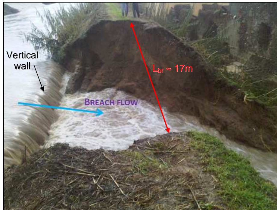
Figure 5.21: Side view of the breach of Ombrone river (Tuscany – Italy) in December 2009.
