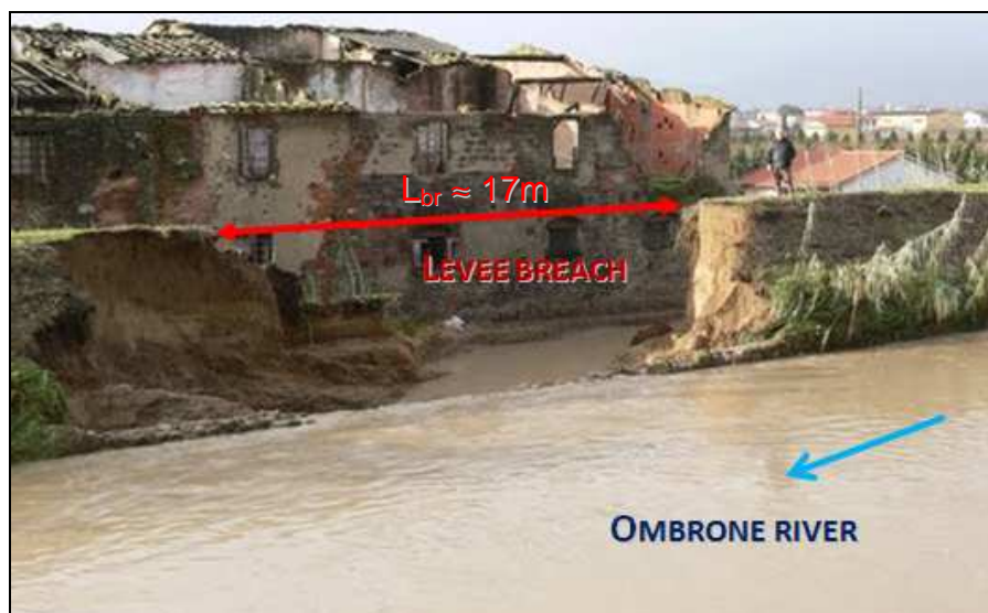
Figure 5.20: Front view of the breach of Ombrone river (Tuscany – Italy) in December 2009.
