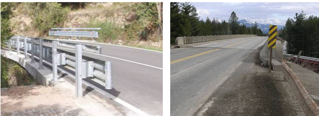
Figure 53: Examples of hazardous safety barrier terminations
