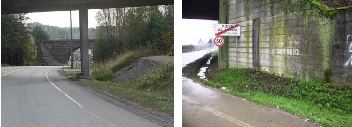
Figure 52: Examples of a hazardous bridge abutment ( left ) and overpass ( right ) (Source: [A.2])
