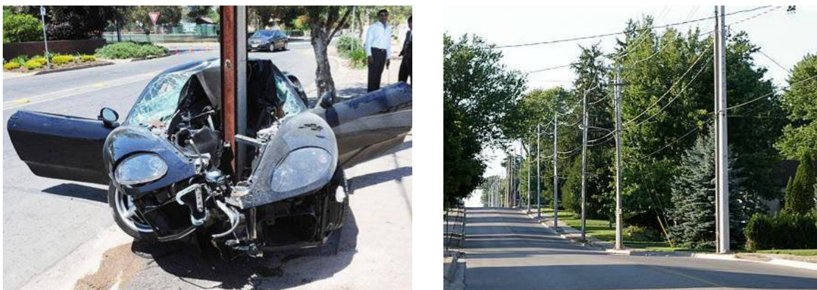
Figure 50: Two examples of hazardous utility poles (Source: [A.51])
