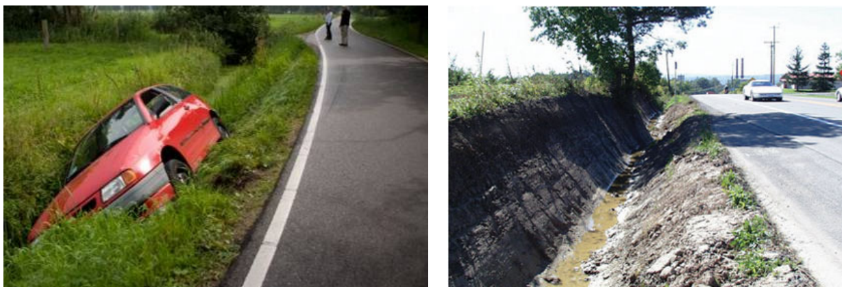
Figure 57: Examples of hazardous roadside ditches (Source: [A.26])
