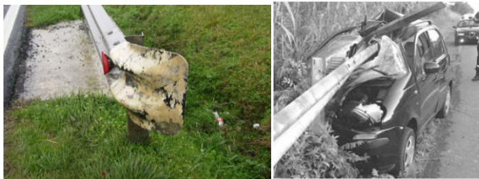
Fig. 2. Unprotected barrier terminals [2]
