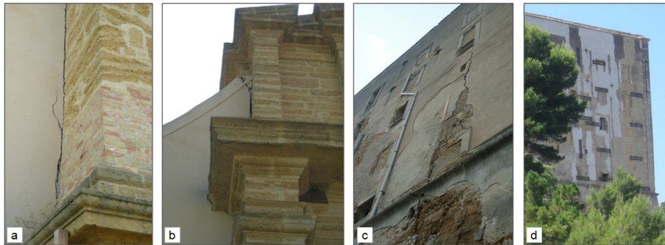
Fig. 6. Example of damages and cracks on the façade of St. Gerlando's Cathedral (a–b) and the Bishop's Seminary (c–d).
