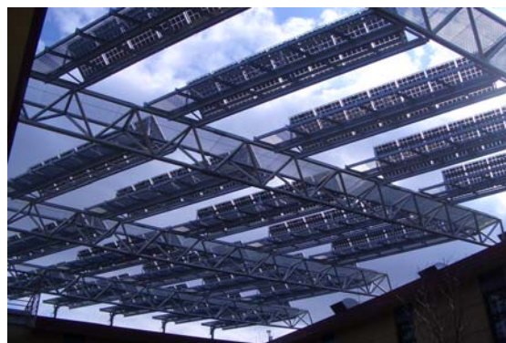
The photovoltaic system
