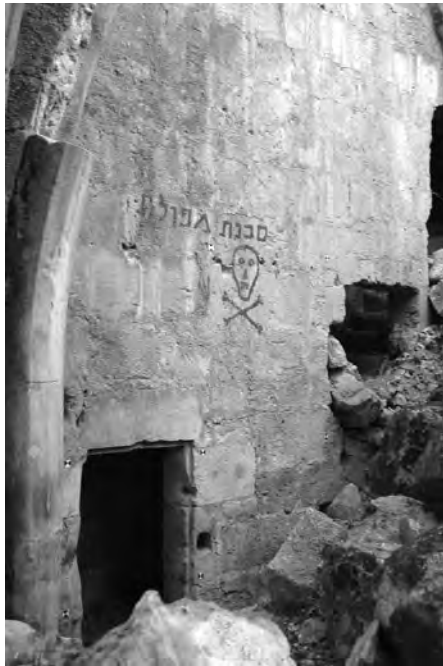
Fig 19 - Guest house: first floor, entrance detail to the stairs that link the second collapsed floor.
