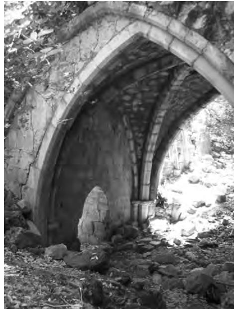
Fig 18 - Guest house: first floor, view from west to the only cross vault still exist.
