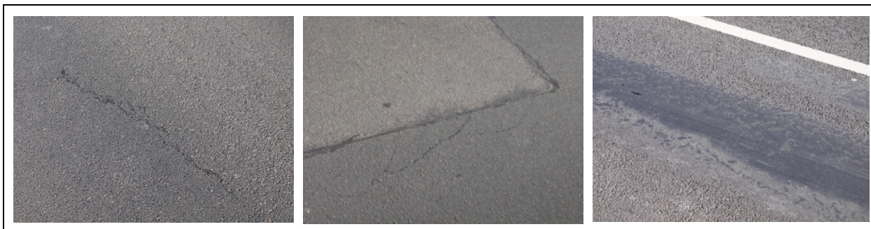
Figure 89: Substance parameter (Network cracks, flick posts, accumulation of bituminous binder).
