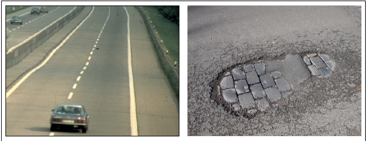
Figure 83: General Unevenness (road surface wave and pothole).
