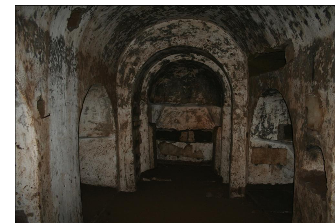
Cubicle Cd where spot microclimate measurements performed in October 2011 highlighted an average CO 2 concentration not less than 4000 ppm.
