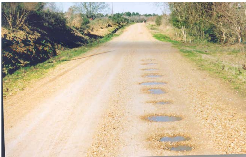
FIGURE 1 Critical roughness on gravel farm road.
