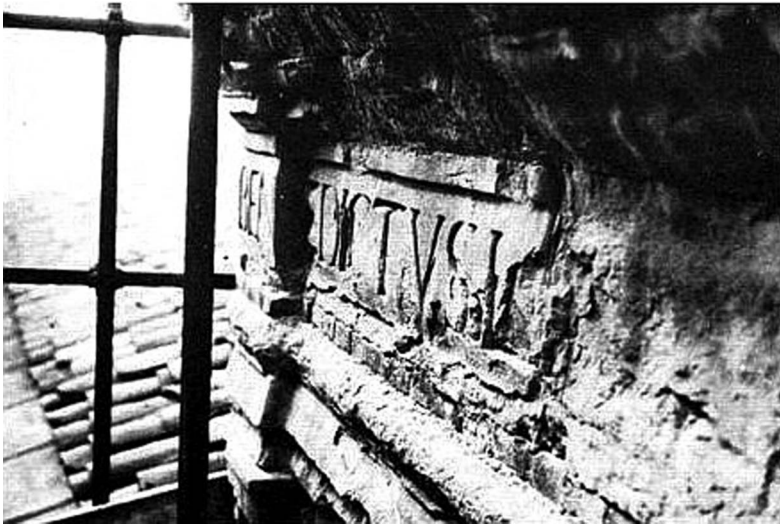
Figure 2. The state of conservation of a portion of facade in 1974.
