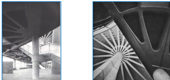
Figure 6. Intrados views of the R/C ribbed slabs of the gallery floors
