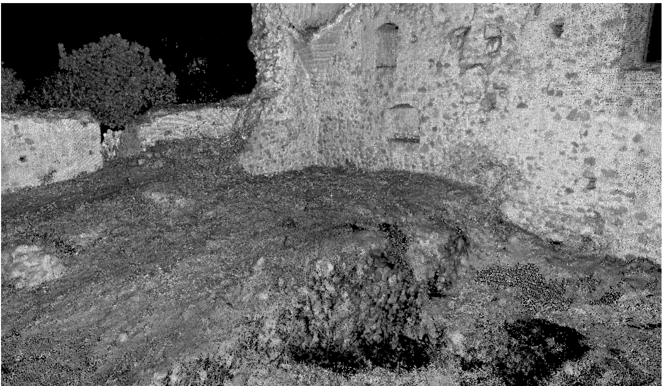
Figure 2. The rooms inside the castle are not accessible at present as they are entirely obstructed by fallen building material (view from the points model surveyed using a laser scanner)
